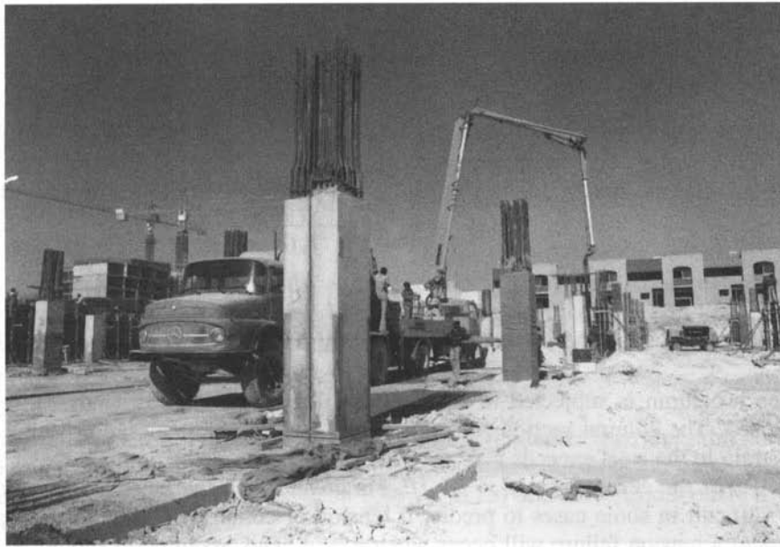
Reinforced concrete tied columns under construction. The two columns are separated by an expansion joint.
