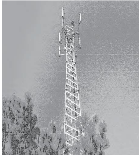
Fig. 5.5 Cell-site antenna tower with various antennas mounted on it
