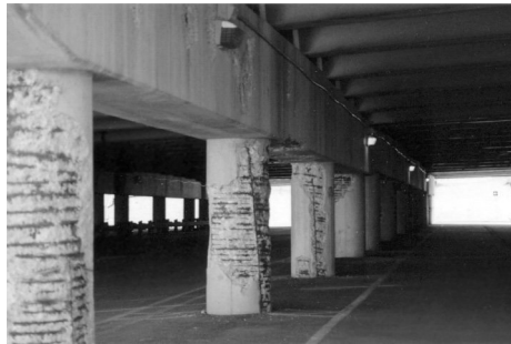
FIGURE 16.12 Deteriorated concrete columns.
