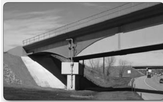
FIGURE 3.24 This drainage system and blocky pier clash with an otherwise attractive overall aesthetic scheme. Union Pacific Railroad Bridge over I-25, Castle Rock, Colorado. (From AASHTO, Bridge Aesthetics Sourcebook , American Association of State Highway and Transportation Officials, Washington, DC, 2010. With permission.)
