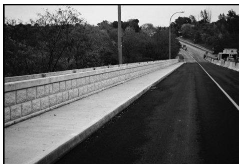
FIGURE 16.27 Deck rehabilitation of Glendale Avenue Bridge.(From ISIS, Design Manual 3: Reinforcing Concrete Structures with Fibre Reinforced Polymers . ISIS Canada, Intelligent Sensing for Innovative Structures, A Canadian Network of Centres of Excellence, University of Manitoba, Winnipeg, Manitoba, Canada, 2007a. With permission.)
