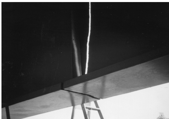
FIGURE 19.3 View of cracked girder of I-79 Bridge at Neville Island in Pittsburgh as an example of a bridge that is sufficiently redundant to avoid collapse despite a fracture of the tension flange and the web.
