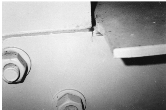
FIGURE 19.9 Close-up view of a crack originating at the termination of a flange on a floorbeam with a “simple” connection to an attachment plate in the Dresbach Bridge in Minnesota. The crack is an indication of an end moment in the simple connection that is not predicted in design.
