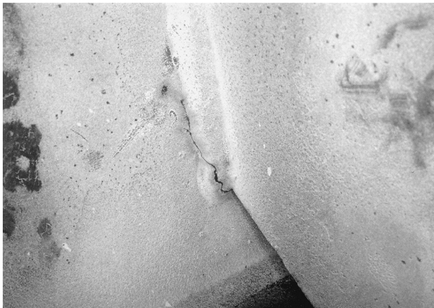
FIGURE 19.7 View of crack in the fillet weld joining the diaphragm connection plate to the web of a box section in the Washington Metro elevated structures. The crack is caused by distortion in the small gap between the bottom of the attachment plate and the box girder flange.
