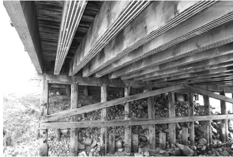
FIGURE 16.16 Tour and Creek Bridge, Manitoba, Canada after strengthening for flexure.
