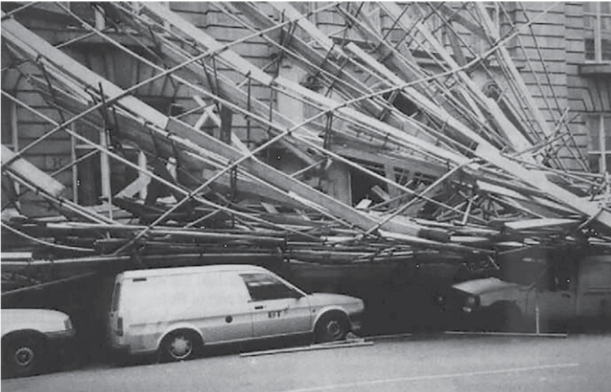
Figure 3.21 Collapse of a scaffolding structure (Courtesy of Mr John Anderson).
