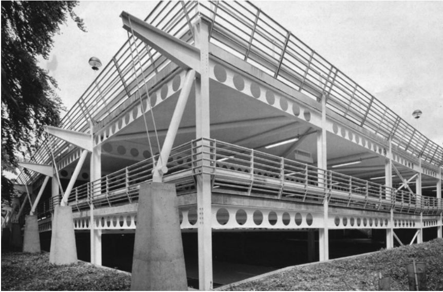
Figure 4.5 Overhangs and tendon forces are used to reduce bending moments and deflections of cellular beams (Courtesy of Mr John Calverley, UK).
