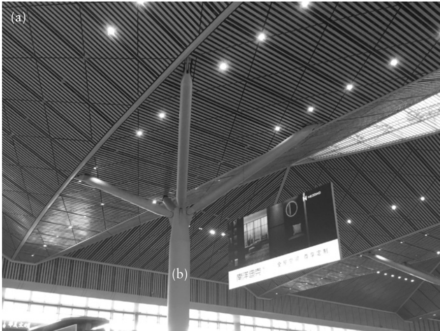
Figure 6.22 The roof supports of the Xi'an North Railway Station, China. (a) Overview of the roof and its supports. (b) A typical Y branch support and overhangs.
